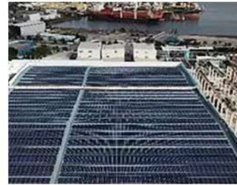
Project Location: Tuas, Singapore Capacity: 1MWp Completion Year: 2017 Type: Metal roof Mounted
