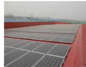
Project Location: Iloilo, Philippines Capacity: 1.9MWp Completion Year: 2016 Type: Metal roof Mounted
