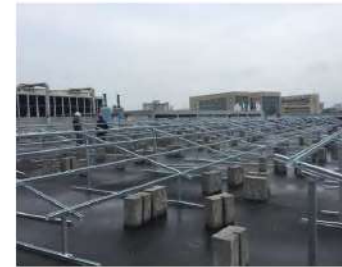
Project Location: Tuas, Singapore Capacity: 1MWp Completion Year: 2017 Type: RC Roof Mounted
