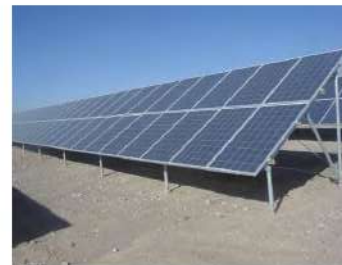
Project Location: Africa Capacity: 1.6MWp Completion Year: 2015 Type: Ground Mounted
