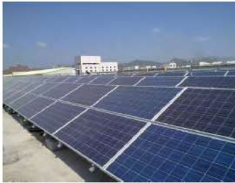
Project Location: Shanghai, China Capacity: 60MWp Completion Year: 2018 Type: Concrete Roof Mounted
