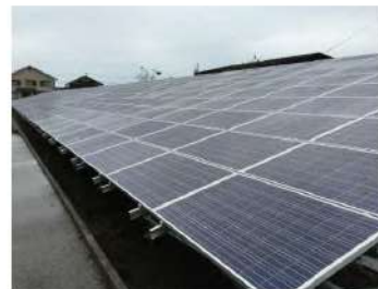
Project Location: Shiga-ken, Japan Capacity: 2MWp Completion Year: 2015 Type: Ground Mounted
