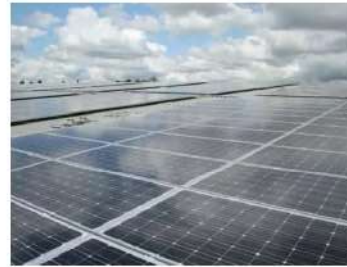
Project Location: Klang, Malaysia Capacity: 426kWp Completion Year: 2016 Type: Metal roof Mounted
