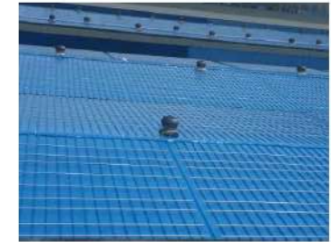
Project Location: Singapore Capacity: 221Wp Completion Year: 2017 Type: Metal roof Mounted
