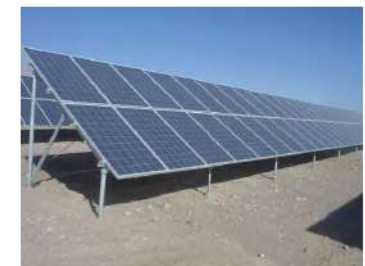
Project Location: USA Capacity: 2.5MWp Completion Year: 2015 Type: Ground Mounted
