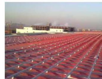
Project Location: Africa Capacity: 1.6MWp Completion Year: 2015 Type: Metal Roof Mounted
