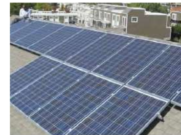
Project Location: USA Capacity: 2.5MWp Completion Year: 2015 Type: RC roof Mounted
